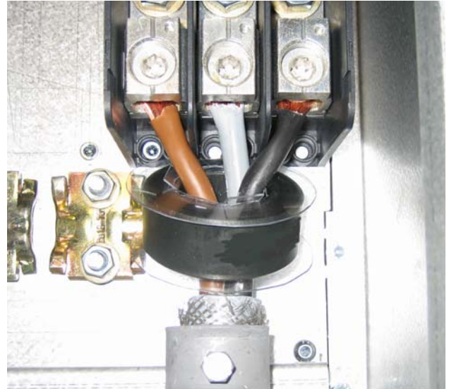
Fig. 49 Ferrite core mounted on the motor cables
